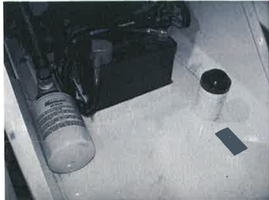
Fig. 25 - Hydraulic Filter and Battery
